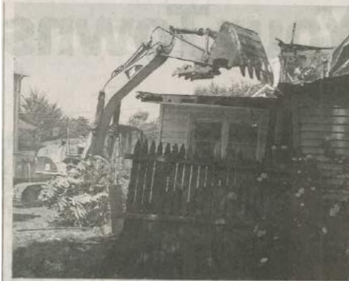
The Orange Housing Authority held a news conference on Thursday announcing the first stage of construction for the expansion of the Dr. Walter G. Alexander Village.
