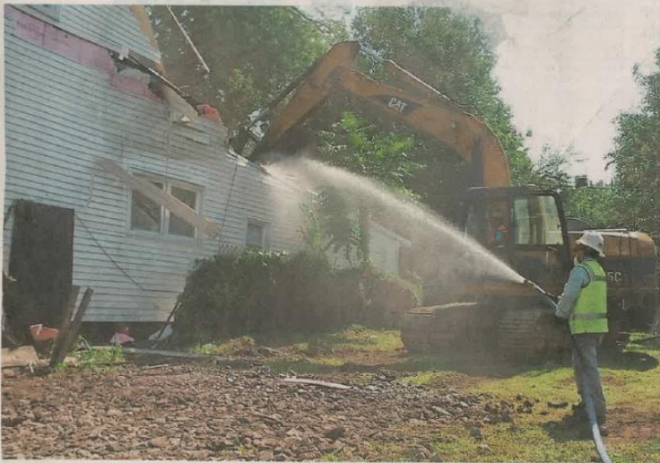
The Orange Housing Authority held a news conference Thursday announcing the first stage of construction for the expansion of the Dr. Walter G. Alexander Village. Demolition also began on Central Place. Patti Sapone/NJ Advance Media for The Star-Ledger
